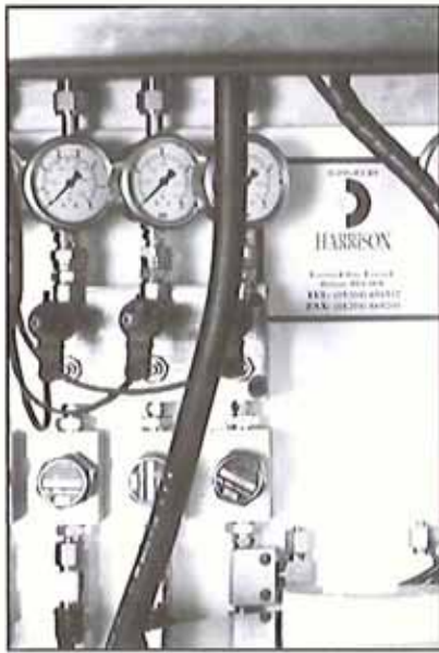
Individual grease filtration and monitoring of each individual grease feed line
